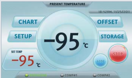
Main Display of Controller
